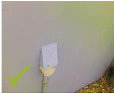
A power outlet has been shielded appropriately.
