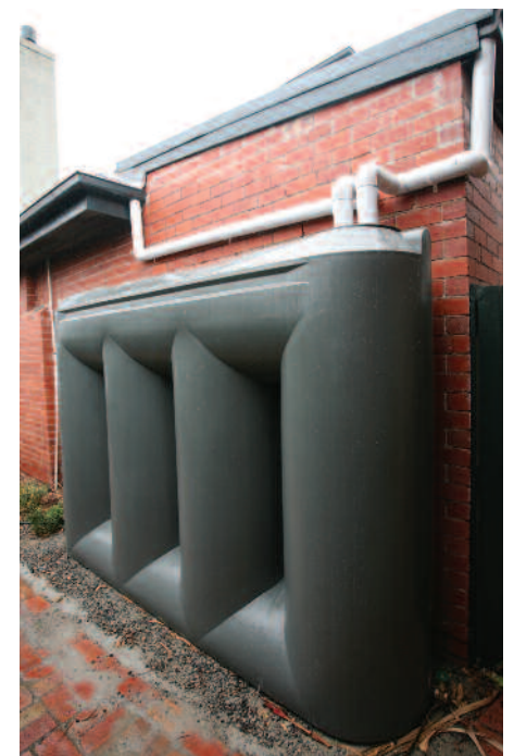
3,000 litre slim line – approx $2,000 inc professionally installed.
